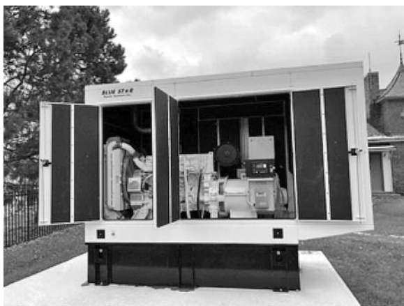
Below: new emergency generator
