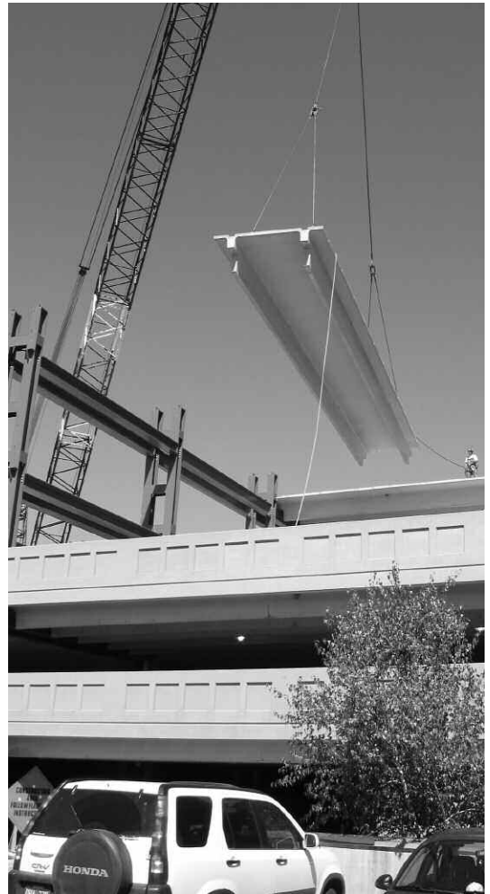
New decks were added to the City's parking garage on Cherry Street.
