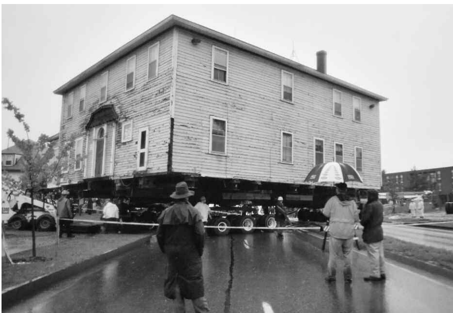
UVM's Johnson House is moved across Main Street to a new site.
