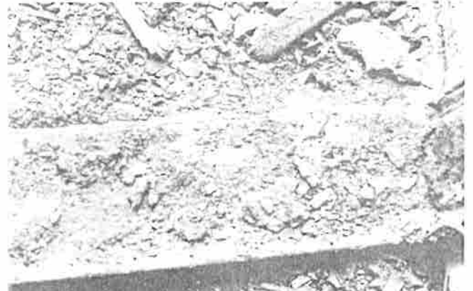
Fig. 6 d. View looking down towards the sill. The subframes appeared very rusted, but were in good condition once debris was vacuumed and surface rust was removed, in place, with chemical compounds. Where necessary, epoxy and steel filler was used to patch depressions in order to make the subframe serviceable again.
