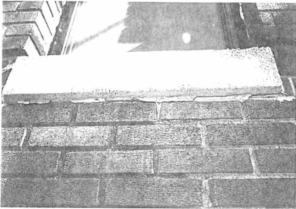
Figure 3 - View of a concrete sill on the exterior of the building. Notice the caulking that was used to patch failed mortar around the sill.
