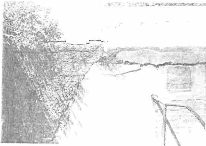
Fig. 6. Battery Fortifications, Ft. Washington, Maryland (1891-97). This unreinforced concrete fortification exhibits several kinds of deterioration: the diagonal structural crack due to uneven settlement, the long horizontal crack at the cold joint, the spalling of the concrete surface coating, and vegetative growth. Photo: Sharon C. Park, AIA.
