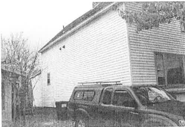
The north elevation has only 1 window, most likely others were removed or covered over.
