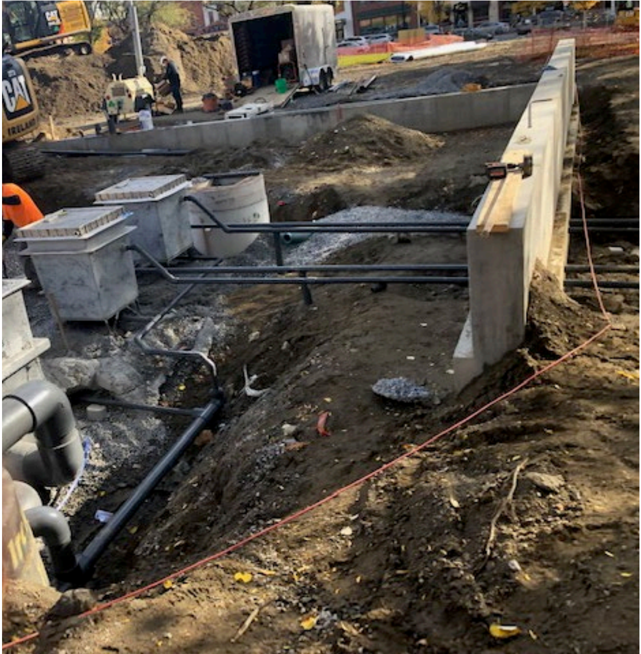
Chemical Tanks Plumbing (below location of Kiosk)
