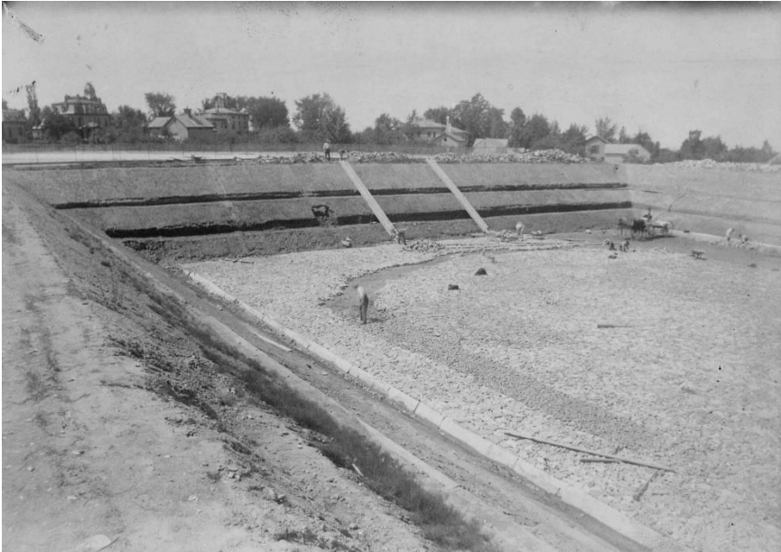
(Left) Digging of our North Storage Reservoir, circa 1868. (Bottom) Relining the same Reservoir in 2015. Note that both Reservoirs were covered in 1981 to protect your drinking water.
