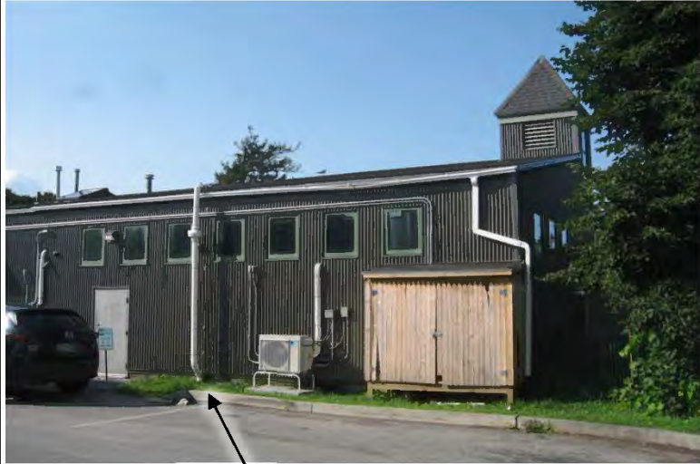
Riser and fan for sub-slab depressurization system
